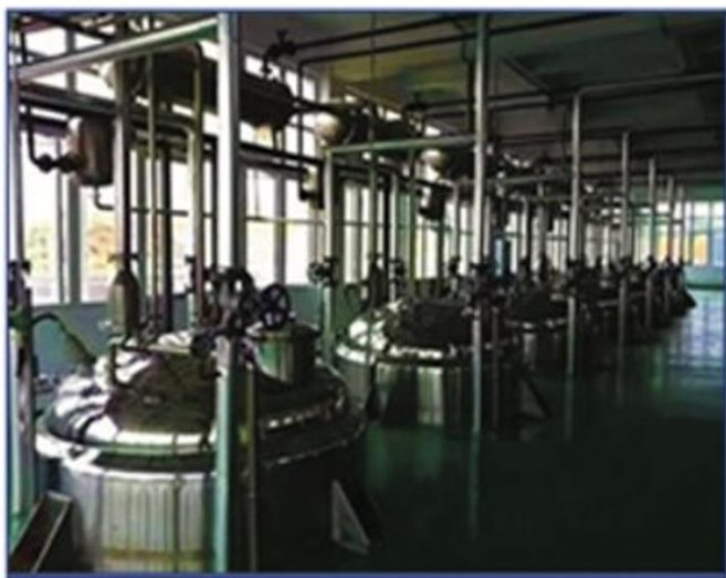
Fluorinated Liquid Production Reactor
